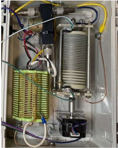
Figure 7 – ATU. On the top left-ish is the relay for switching in/out the 160m inductor. The 80m inductor can be seen on the bottom left and the 160m inductor on the right.
